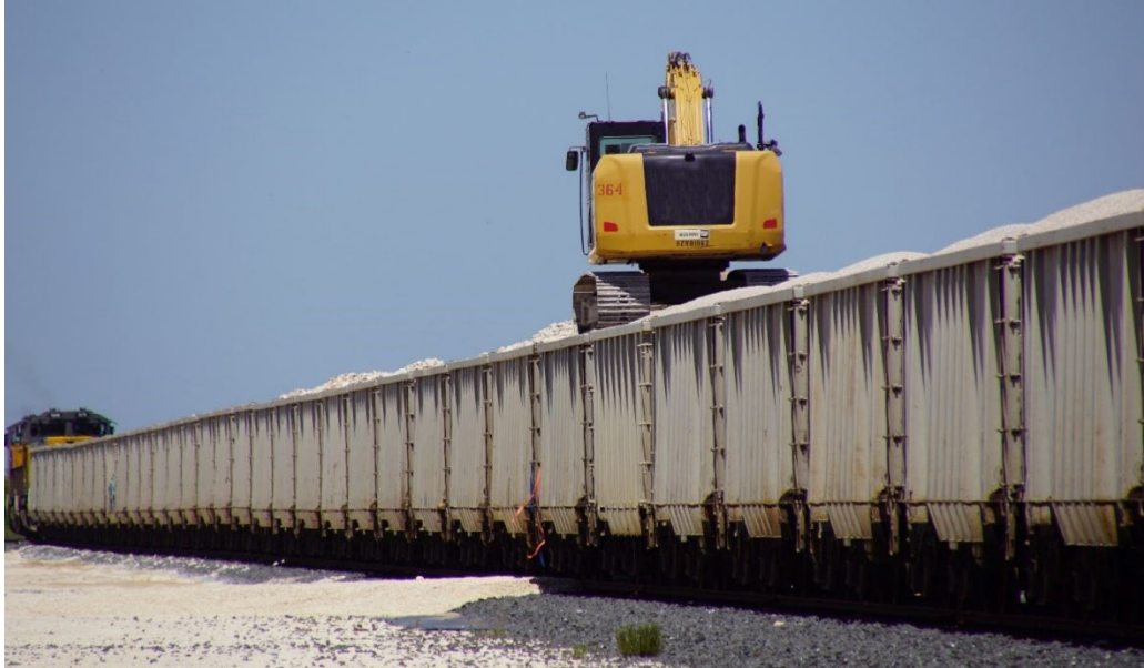
PHOTO CUTLINE: An excavator unloads Vulcan Materials Company's first rail shipment of bulk aggregate to Port Freeport's Parcel 14.
